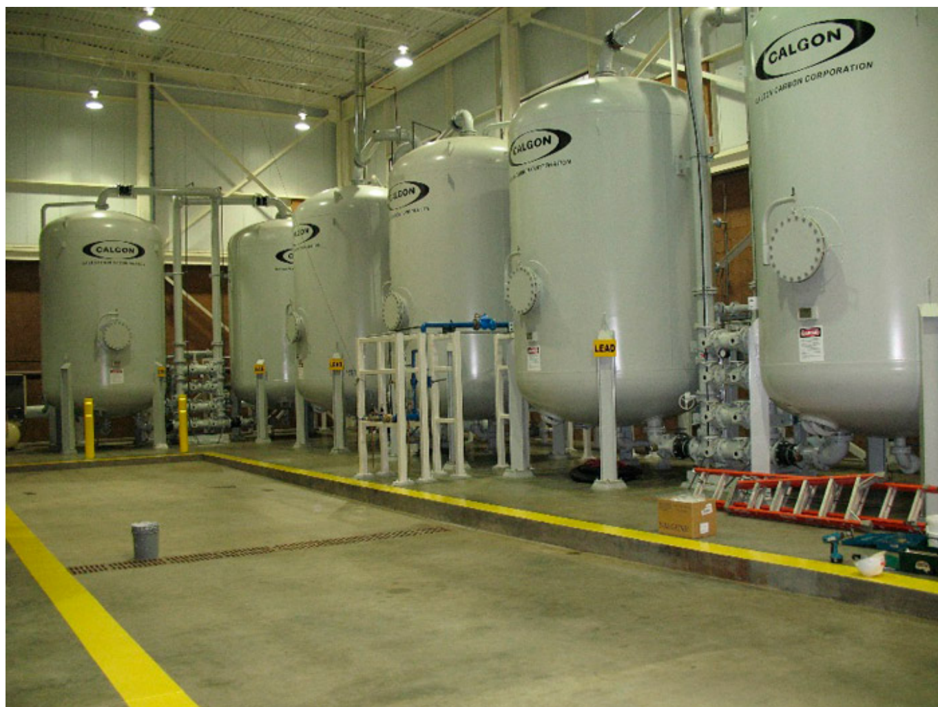
Figure 15-6. GAC treatment system, Oakdale, MN.
